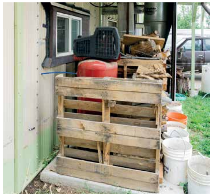
Locating the compressor and dust collector outside of the workshop will reduce the noise and dust problems significantly inside
