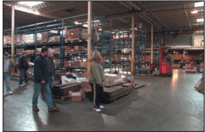
Fig. 10 With the expansive space that is available, it is a lot of work just getting the shelving erected and the remodeling done.
